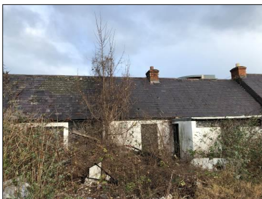
Plate 6.3 - Rear view of derelict cottages along N11.
