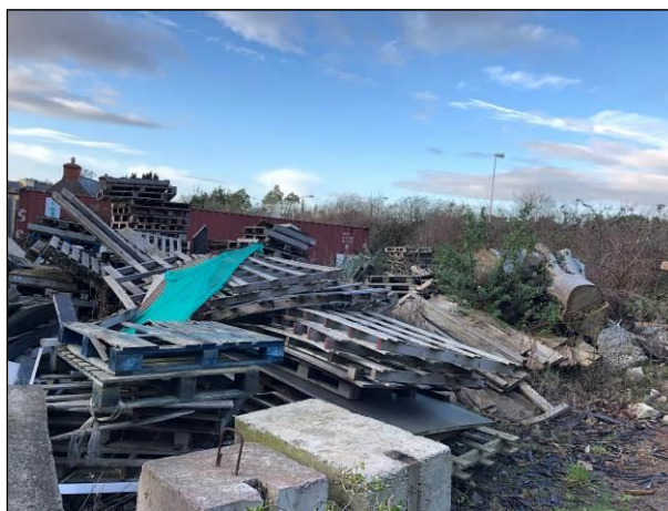
Plate 6.6 - Example of building waste and construction materials on site.
